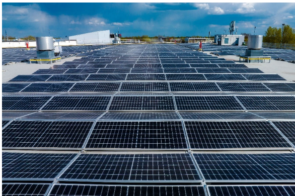
(a) roof-mounted BAPV system
