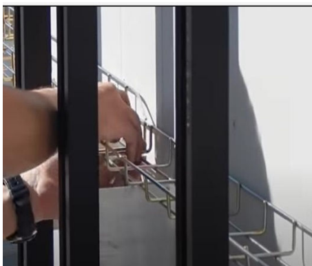
(a) open cable trays (photo courtesy of Onyx Solar)
